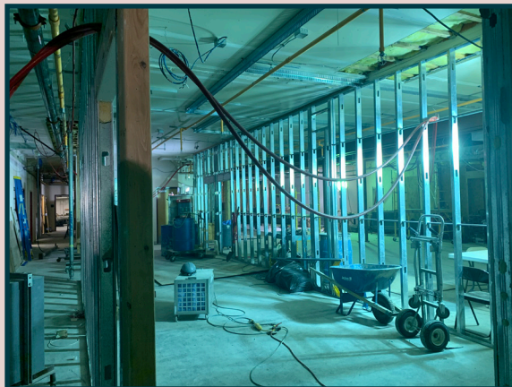
Work on the south wing of the Poldine Carlo Building started last fall. The construction includes five new Head Start classrooms to be completed June 2020.
